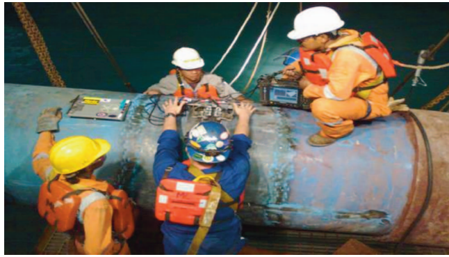
Figure 1. On the Manifa pipeline project, VML needed to specify a welding process and materials that would work on heavy-duty pipe and in a sour environment, while keeping the project running at a productive pace, on time and on budget.
