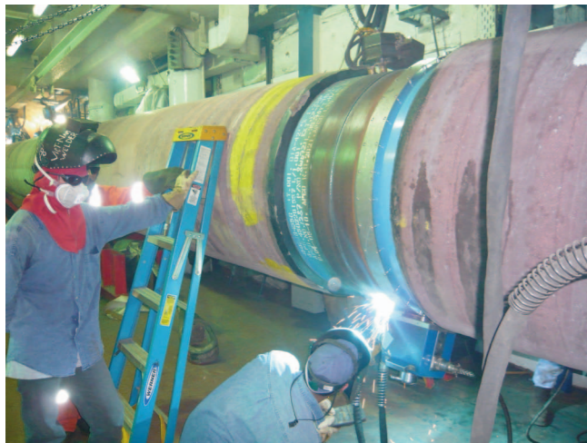
Figure 2. While working on the pipeline, welders were able to achieve precise wire placement. The cast and pitch of the spooled wire was maintained from start to finish. Once placed, it did not wander from the joint.
